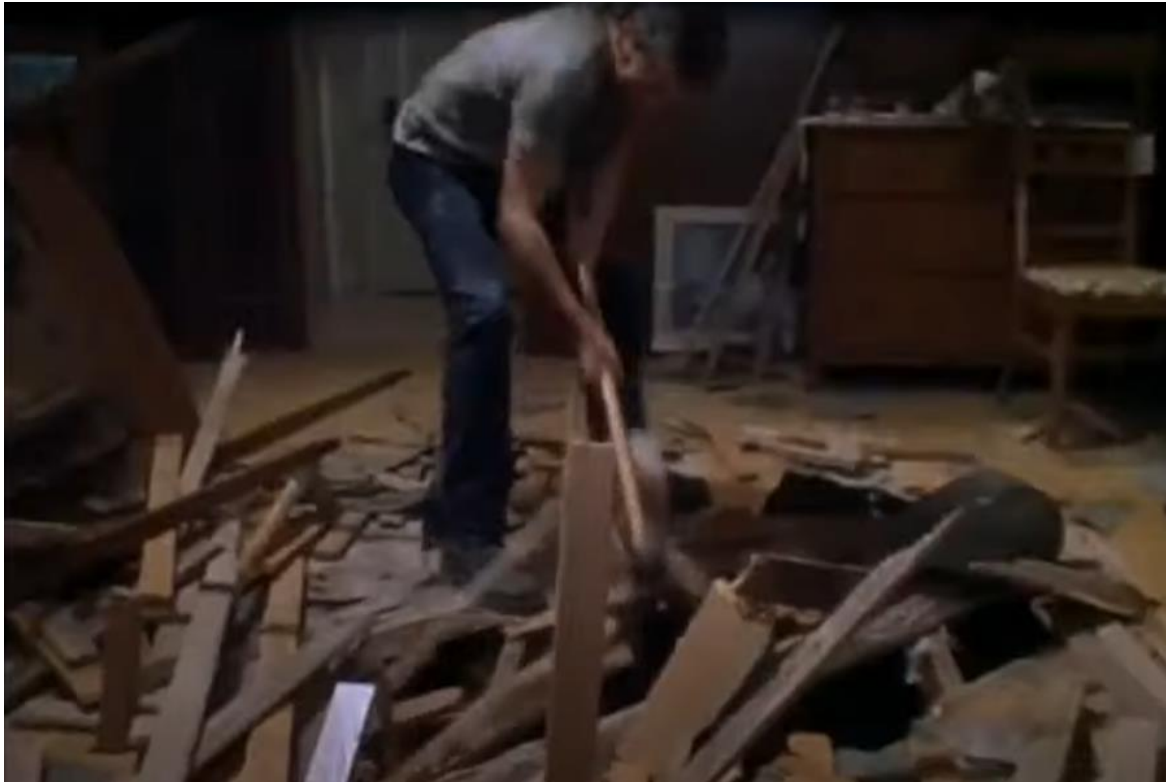
Figure 41: The hole in the dining room floor.
