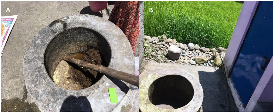
Figure 2.6: Two cow dung and food waste biogas inlets. (A) shows the inlet with cow dung prior to users mixing with water and moving a stone that blocks the inlet pipe to the digester so the liquid mix can fall via gravity into the digester, (B) shows an empty cow dung and food waste inlet next to the toilet (blue door) and rice field behind the house, the slurry exits the digester and flows freely into the rice fields or can be composted first.
