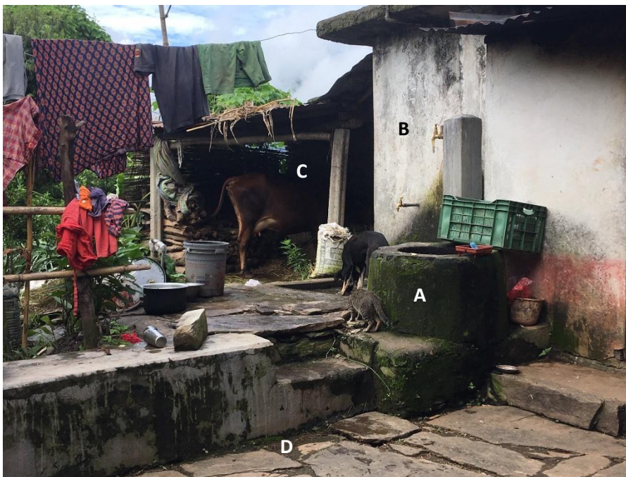
Figure 2.5: TLAD in a rural household in Nepal. The components of the system are as follows; Cow dung and food waste inlet (A) Toilet (B) Animal holding close to house and digester (C) the main TLAD digester dome is situated underground (D).
