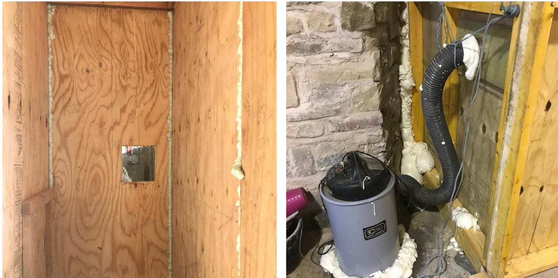
Figure 5.4. Left: the panels, sealed with foam. Right: The installation of the dust/air extractor and the discrepancies between the scribed chamber and stone wall, filled with expanding foam.
