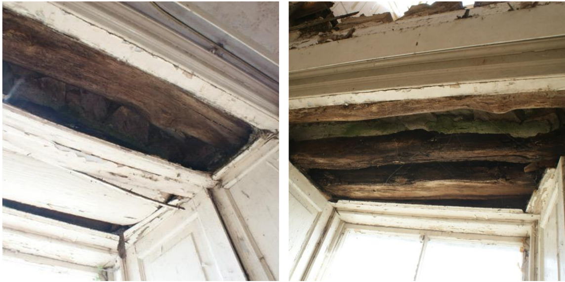
Figure 4.27. Decayed timber safe lintels.
