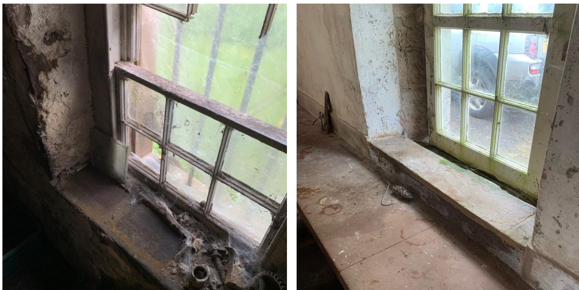
Figure 4.3. Left: Newmills, Resolis, the Black Isle, Ross shire. Right: dairy, Thornhill, Dumfries and Galloway. Non-residential building with full wall thickness below the sill demonstrating the importance of internal light, with little requirement for view.
