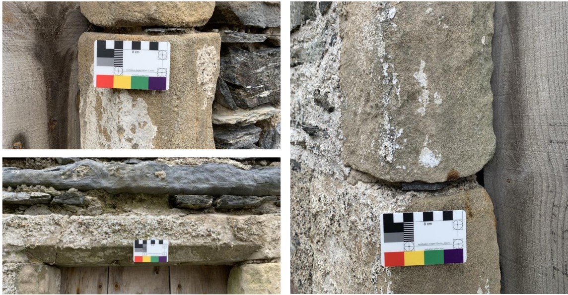
Figure 2.26. Harbour building Portsoy. Harl approaching the chamfer then folding around as fine plaster and limewash.
