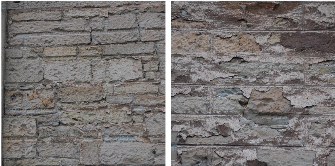
Figure 2.58. Adam's perpendicular and horizontal chasing of the wall surface, subsequently overlain with a thin, single coat, undulating plaster.
