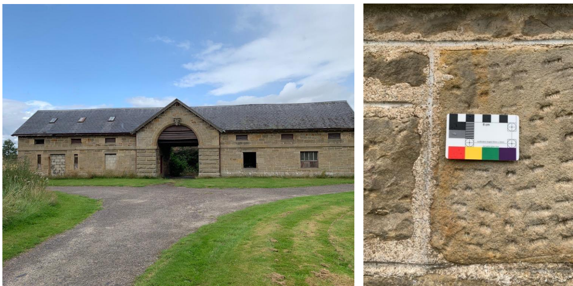
Figure 2.64. Lindores, Morayshire. The formal front (facing the house) with squared rusticated ashlar, lined out and white lined pointing.
