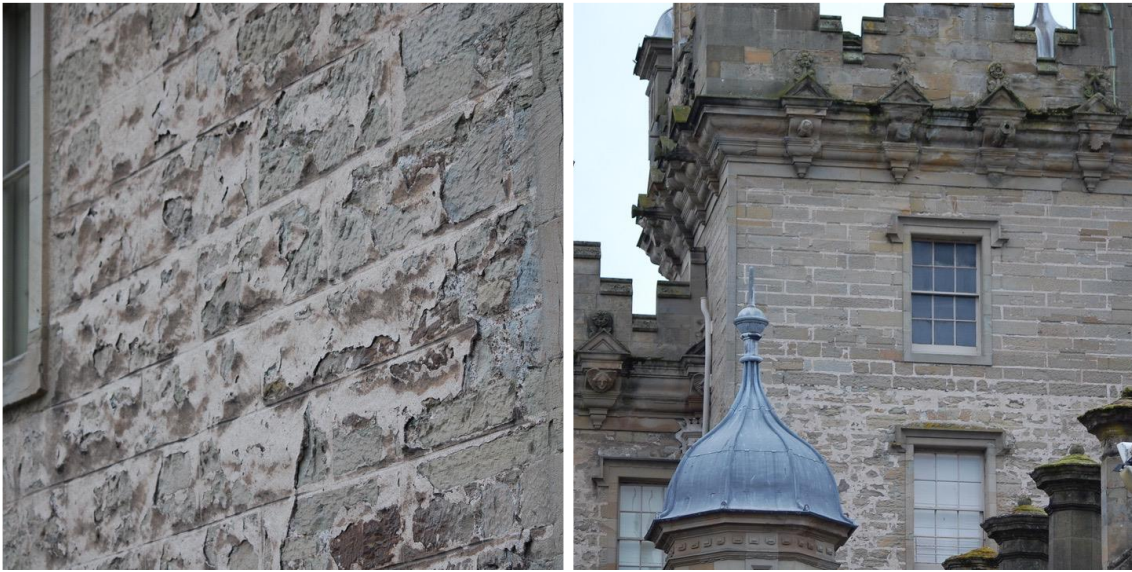
Figure 2.61. Left: decayed fully ruled out plaster, Adam, c.1721. Right: top of the tower, Playfair's work of c.1837. Evenly coursed, pointed and ruled out. Lower tower, Adam's work c.1723. Randomly coursed with fading plaster. This relationship corresponds with Playfair's watercolour scheme in Figure 2.55.
