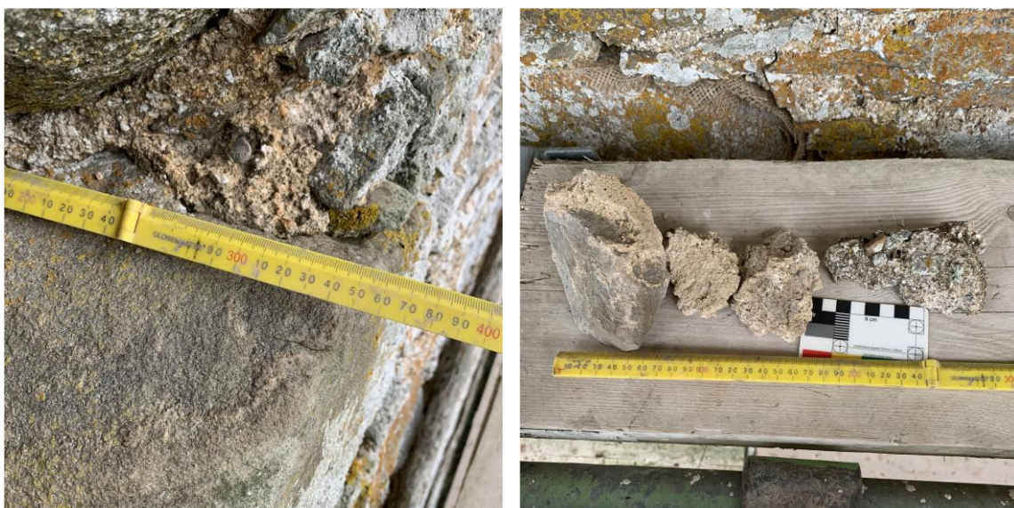
Figure 3.22. Sample FT006 ABC core, bedding and harl locations of mortar on the west elevation Main Tower.
