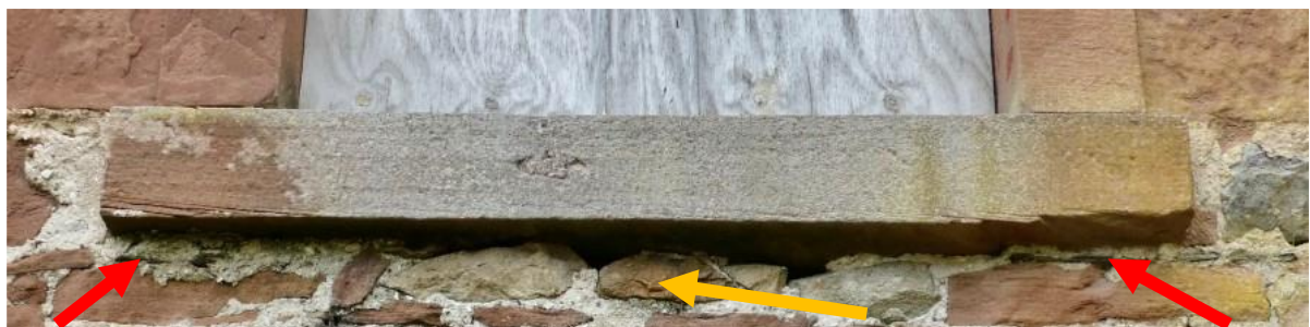
Figure 4.10. The sill placed on pads marked in red either side of the opening and the masonry below left low marked in yellow or added retrospectively.
