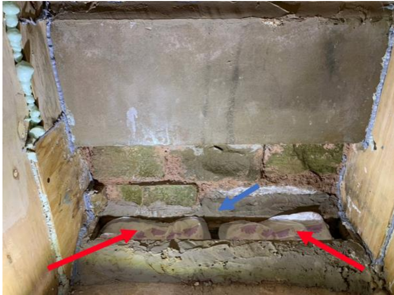
Figure 5.8. The trough permanently fixed with water tabling. The pads in place and joints in the chamber sealed. Red arrows indicate the mats: blue arrows indicate the water tabling.
