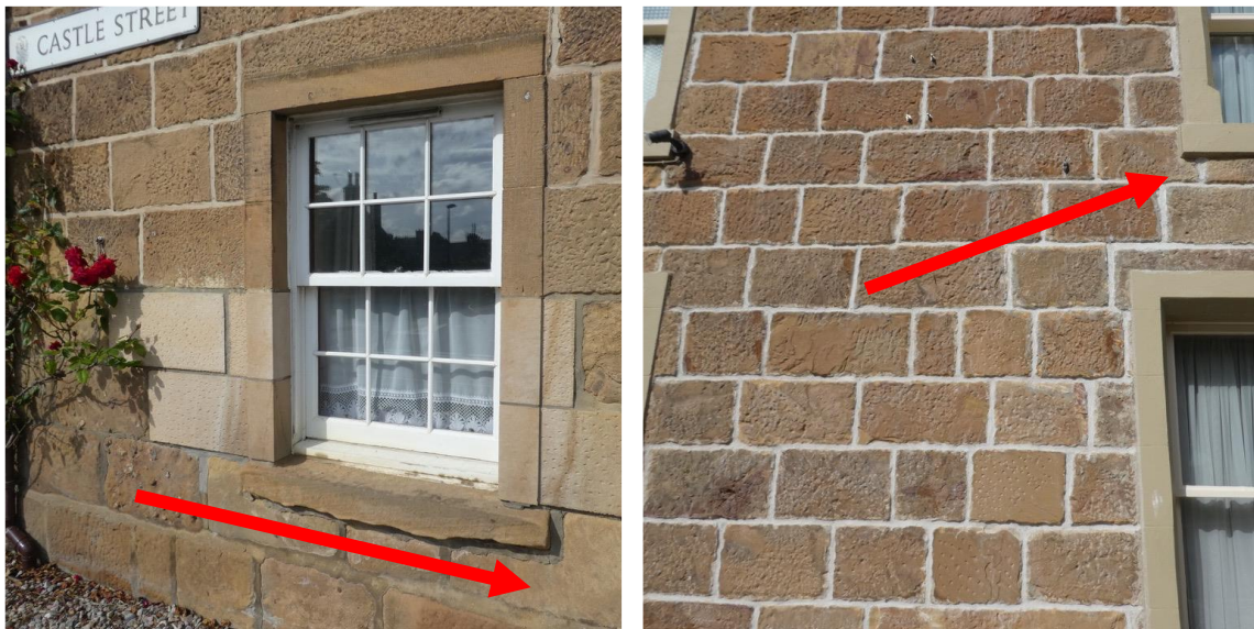
Figure 4.11. The sill placed on pads marked in red either side of the opening and the masonry below left low marked in yellow or added retrospectively.
