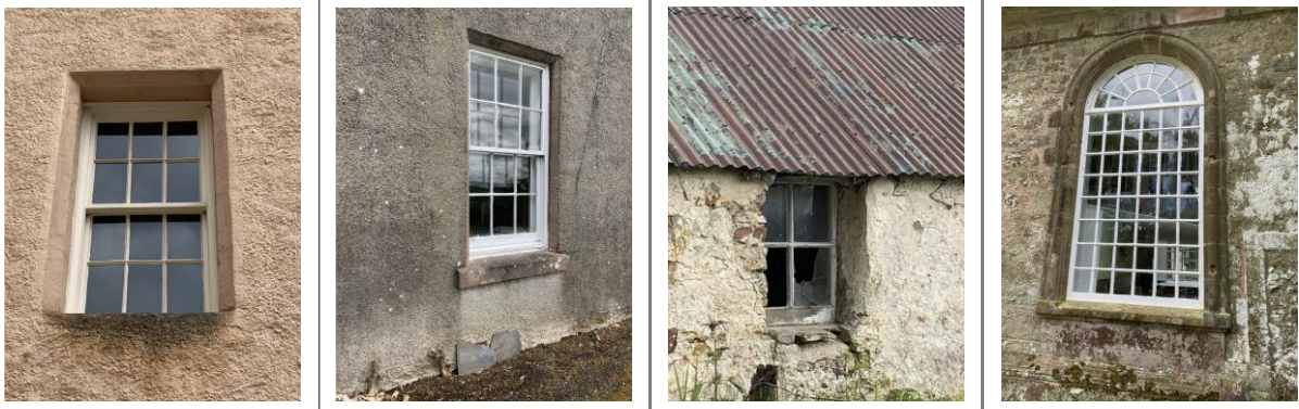
Figure 2.50. Rainwater discharge from glass onto the area below the window: an area of diminished thickness.
