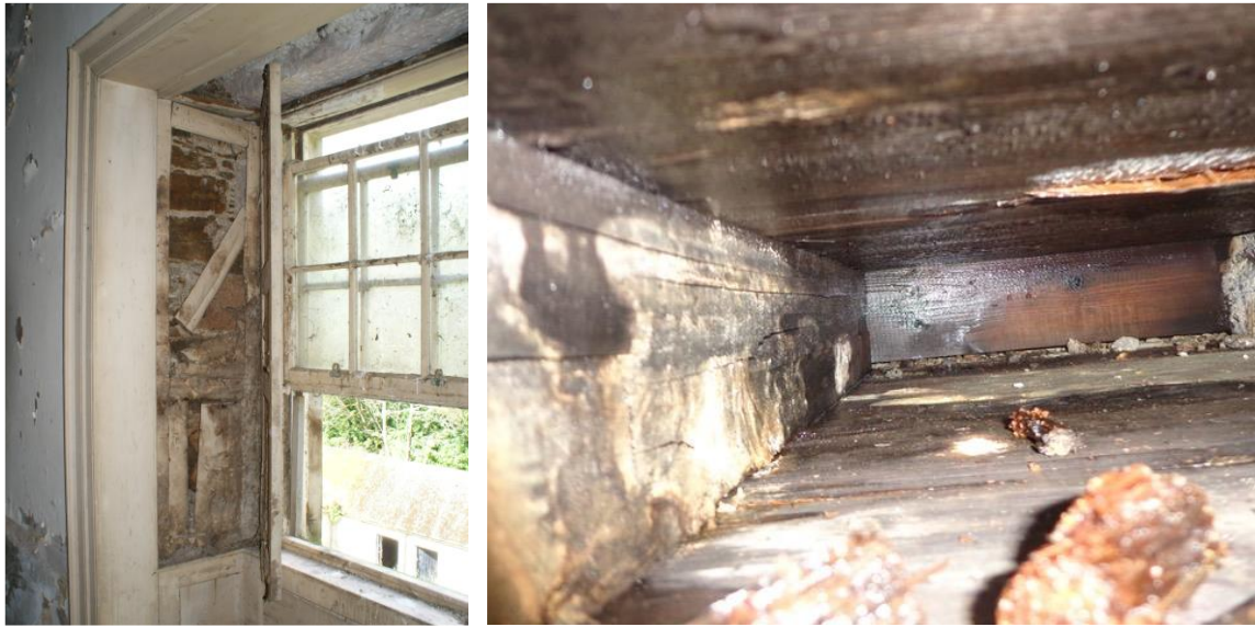
Figure 4.29. Left: window shutters removed revealing damp and decay. Right: In between the floor joists above the window, saturated and much of the water running down the ingoes wetting behind the shutters.
