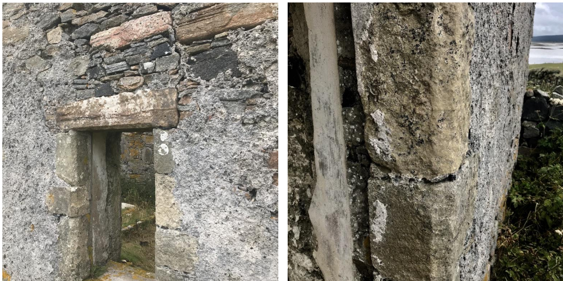
Figure 2.25. Old Vallay House, Uist. Harl approaching the chamfered margin. This then folded around the detail as a finer plaster, as evidenced by the remains in the more sheltered window opening.
