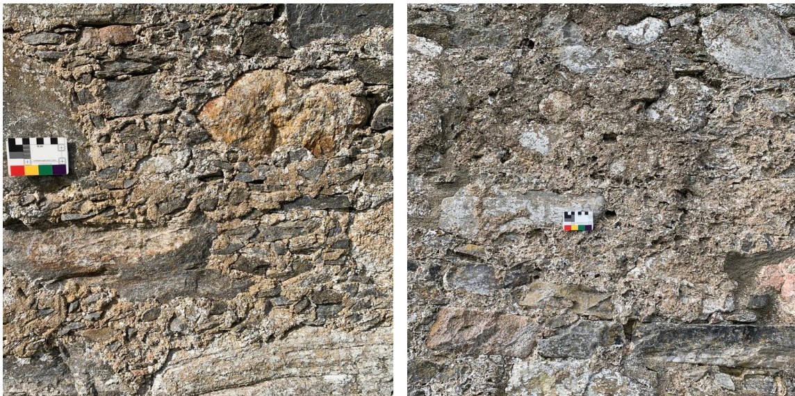
Figure 3.6. The Ruthven Barracks: Left, the Stable block, NE elevation with no remaining evidence of harl or plaster. Right, the Main Barrack block, NE elevation showing extensive harl remains contiguous with the joints, leaving the high points of the stone exposed.
