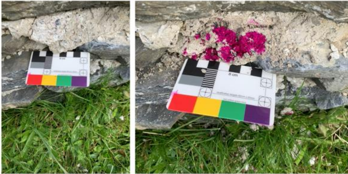
Figure 3.56. SW exposed bare wall surface. Left: Far left the undisturbed surface and right sub-surface sprayed with phenolphthalein with a carbonated depth of <13 mm. Right the uncarbonated mortar > 13 mm.
