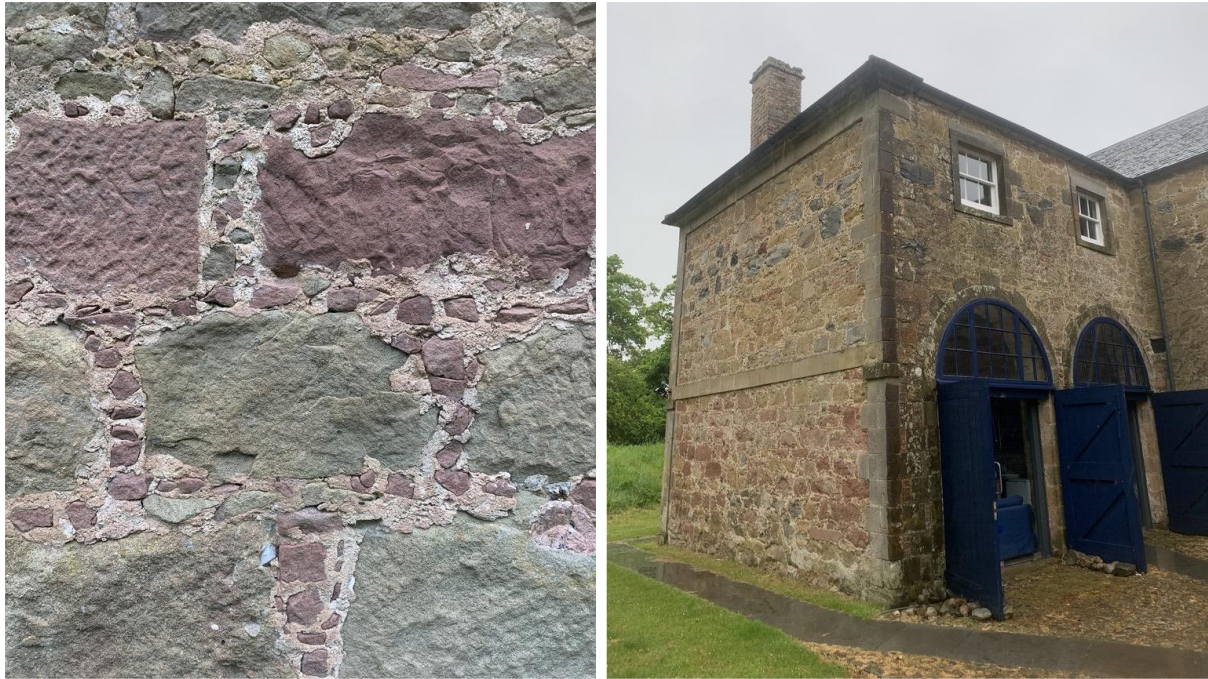
Figure 3.5. Cromarty House Stable Block c. 1785, Cromarty, Ross shire. In this example the joints between the stone survive well due to the cherry-cocking/galleting but the remains of the post-construction harl are scant.
