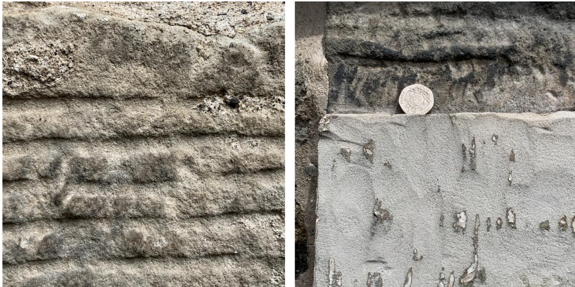
Figure 2.16. Dalgleish Court. Left: broached masonry with extant harl. Right: raised margin, cleaned with an angle grinder yet still retaining traces of limewash.
