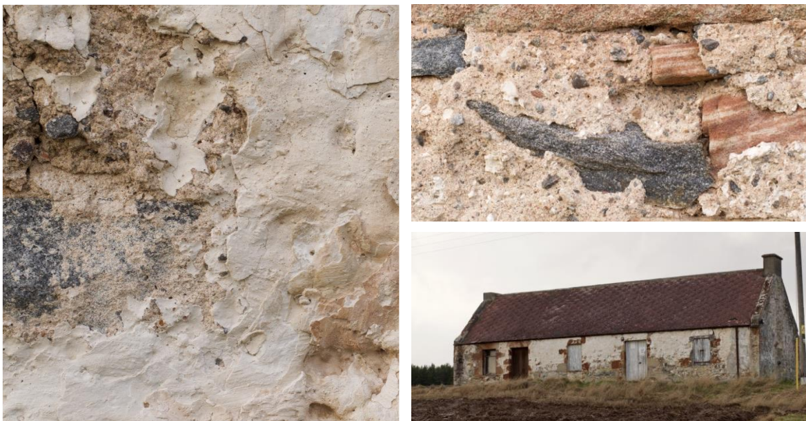
Figure 2.9. Tulloch Cottage, Munloch, Ross Shire. Left: multilayering limewash. Right: an exposed area where harl and limewash had graded away.
