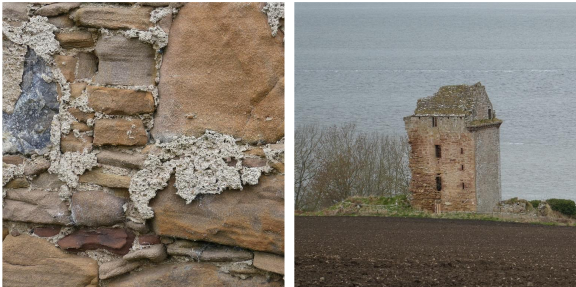
Figure 3.11. Castle Craig, c.1561 Ross shire. Mortar extruded from the joints surviving at the expense of the surrounding sandstone.
