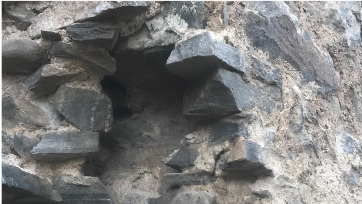
Figure 3.30. The location of sample RB003. The wall core has washed away the majority of the building mortar. In contrast, the wall face retains large areas of harl.
