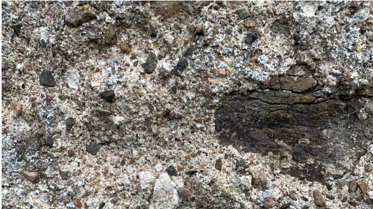
Figure 2.4. Grading away \text{CaCO}_3 / \text{Ca(OH)}_2 exposing angular and sub-angular lithic aggregates embedded in the mortar.
