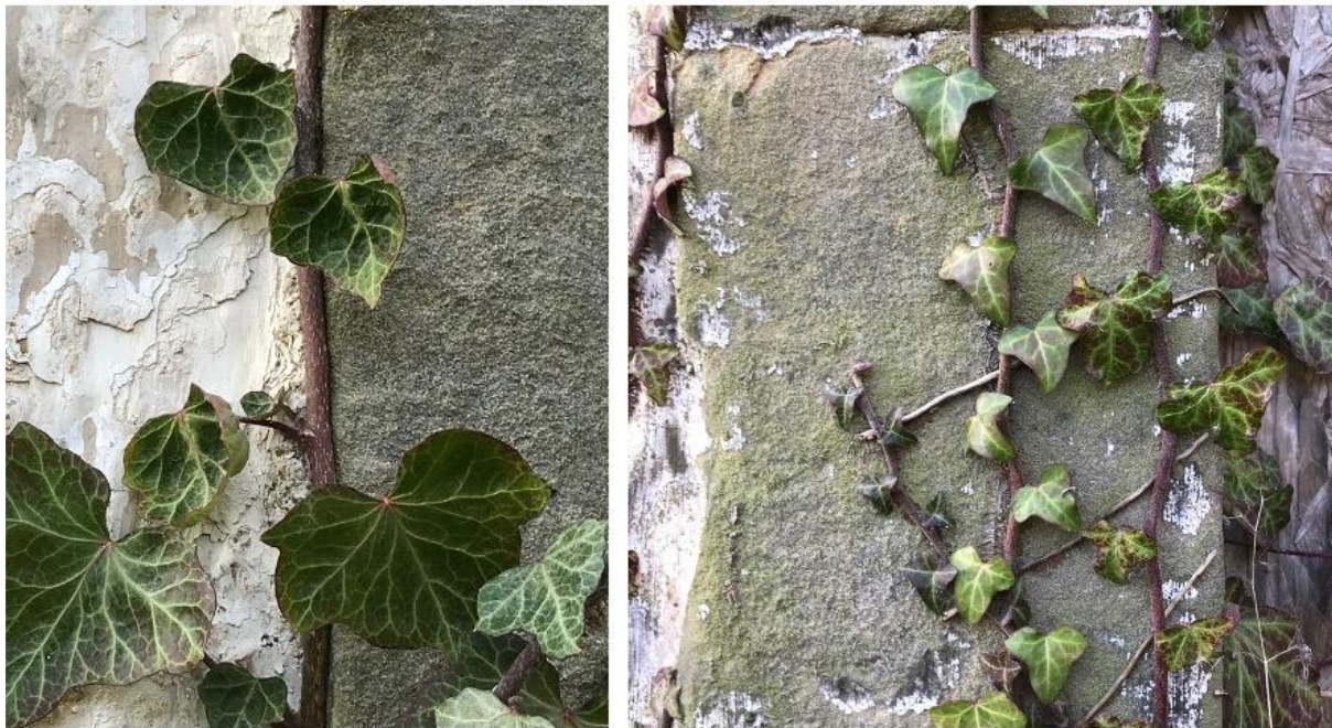
Figure 2.27. The Old School House, Charlestown, Fife. Multi-layers of limewash on the harl with traces still clinging to the raised margins.
