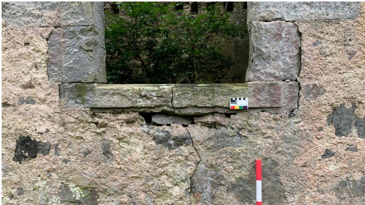
Figure 4.12. The sill joint not in compression, gives way when there is deflection. Note the cracks on each side of the window opening.
