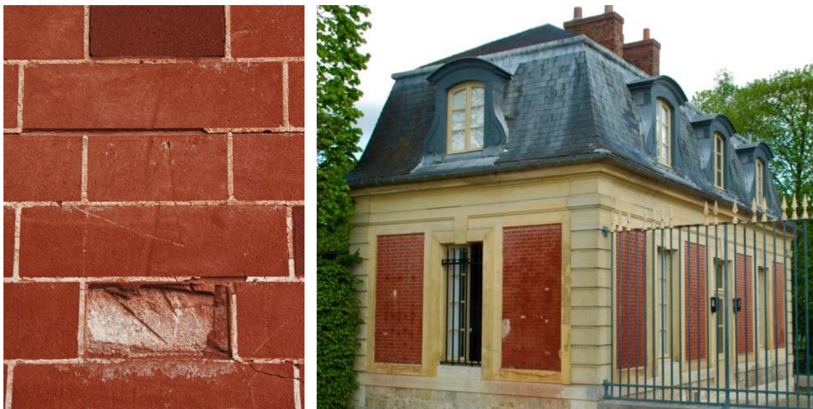
Figure 6.15. The gate lodge from the garden to the alley that leads to Grand Trianon, Versailles. Common brickwork, overlain with plaster, ruled out and white lined to accurately represent fine work. Image credit, Brian Pfeiffer.
