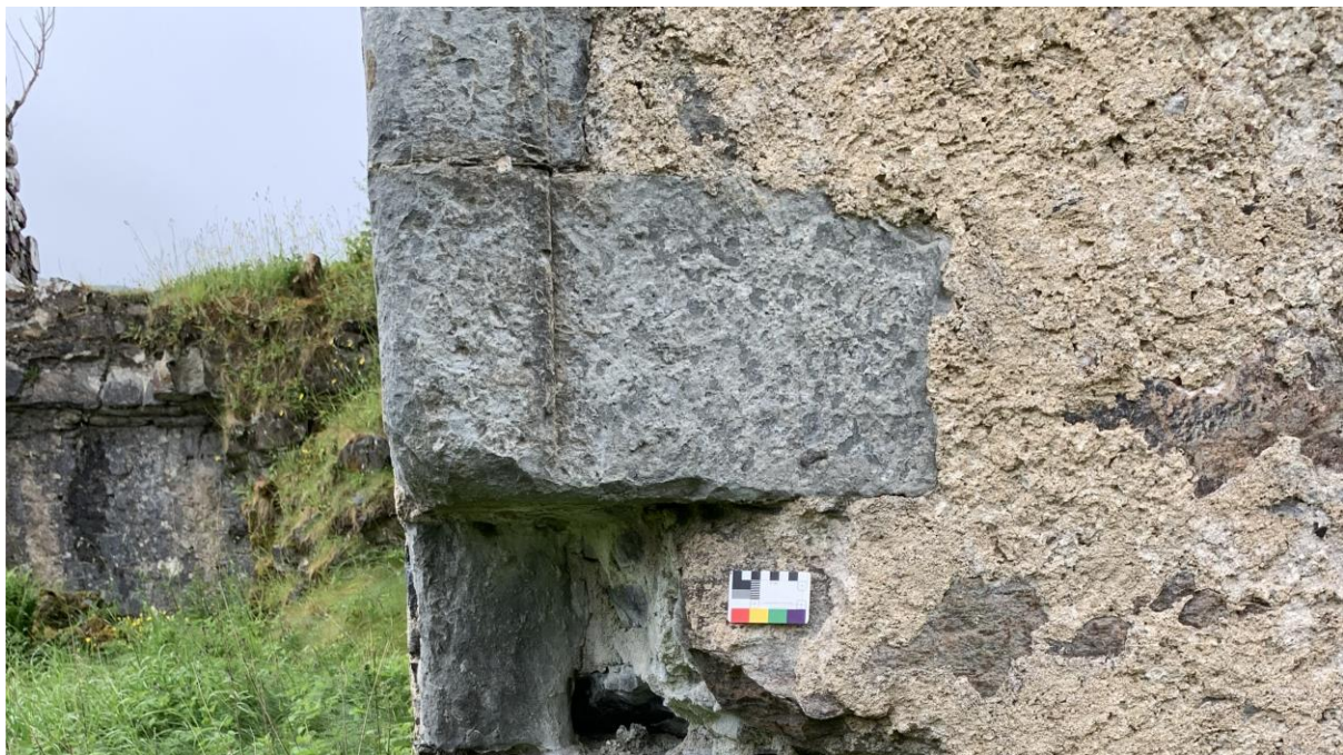
Figure 3.31. Stone robbing undercuts the wall and directs water into the core. Note the green/blue leaching of the limestone quoins.
