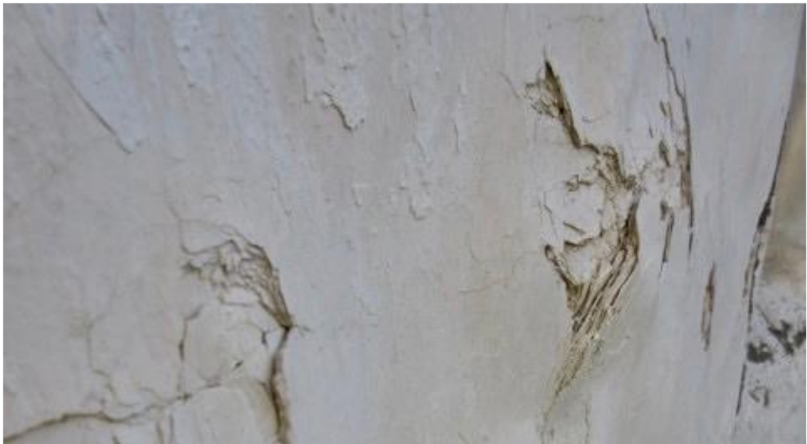
Figure 5.18. Relict multi-layered limewash observed during the survey at Coshoggle Farm, Thornhill, Dumfries and Galloway.
