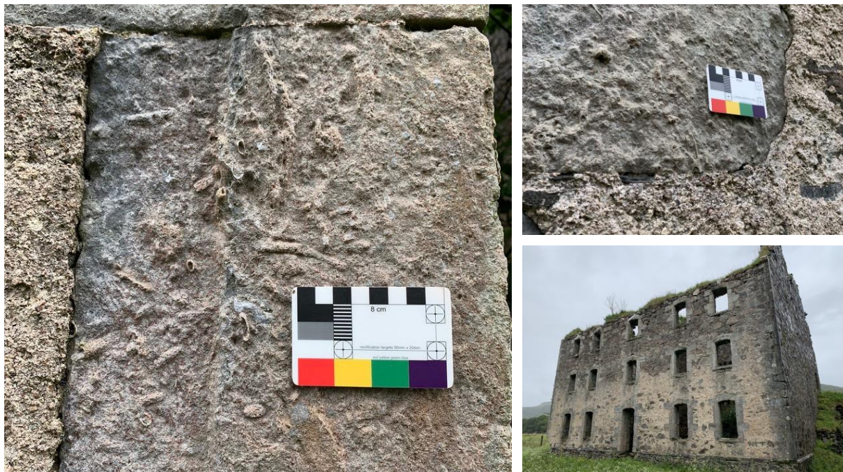
Figure 3.12. The Bernera Barracks, c.1723 Glenelg. Weathered limestone, decaying while the harl remains robust.
