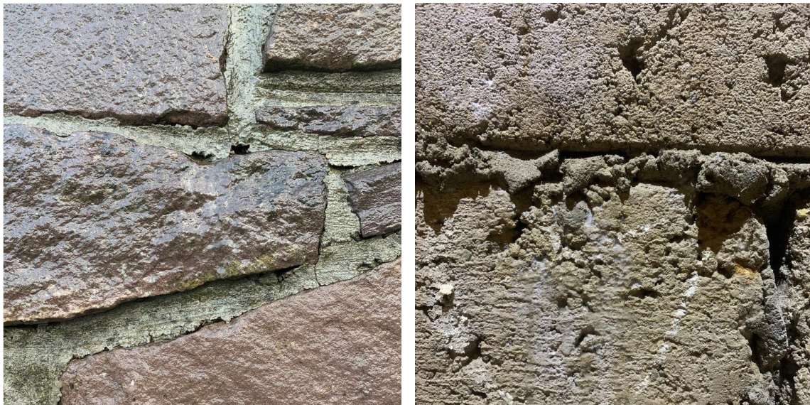
Figure 4.35. Left showing the cracking in cement pointing; Right showing water rivulets running down a cladding of internal blockwork.
