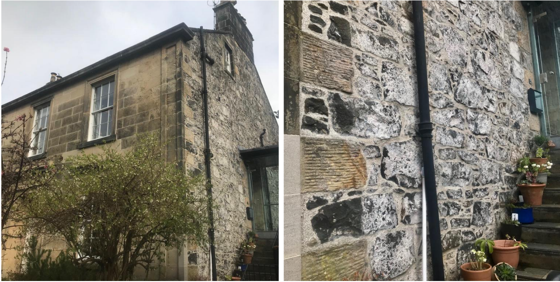
Figure 2.17. Irvine Place, Stirling. Ashlar front, basalt gable and rear elevations with harl extant on the surface of both masonry components.
