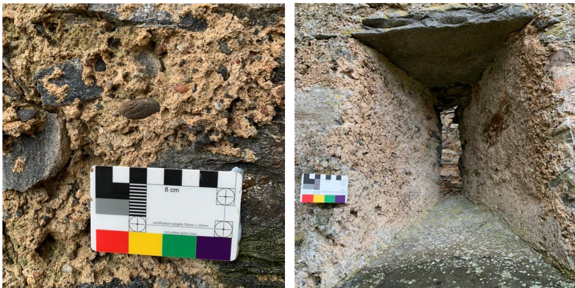
Figure 3.32. Left: shows the external wall face of the S.W. elevation and binder dissolution. Right: the S.W. elevation gun loop, the same mortar but in a sheltered location, retaining binder.
