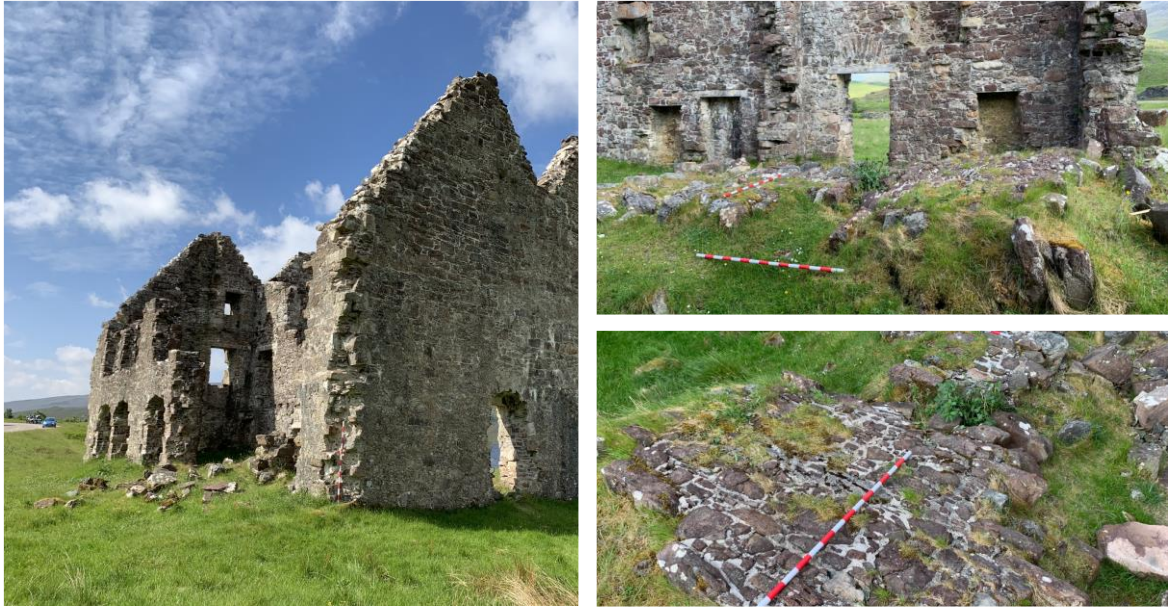
Figure 4.22. Calda House, Sutherland, early 18 th c. showing the collapse of panels of masonry, severed at the insubstantial ties.
