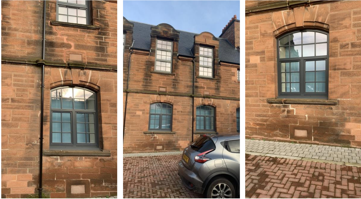
Figure 2.42. Structural issues in and around windows, Perth c.1900.
