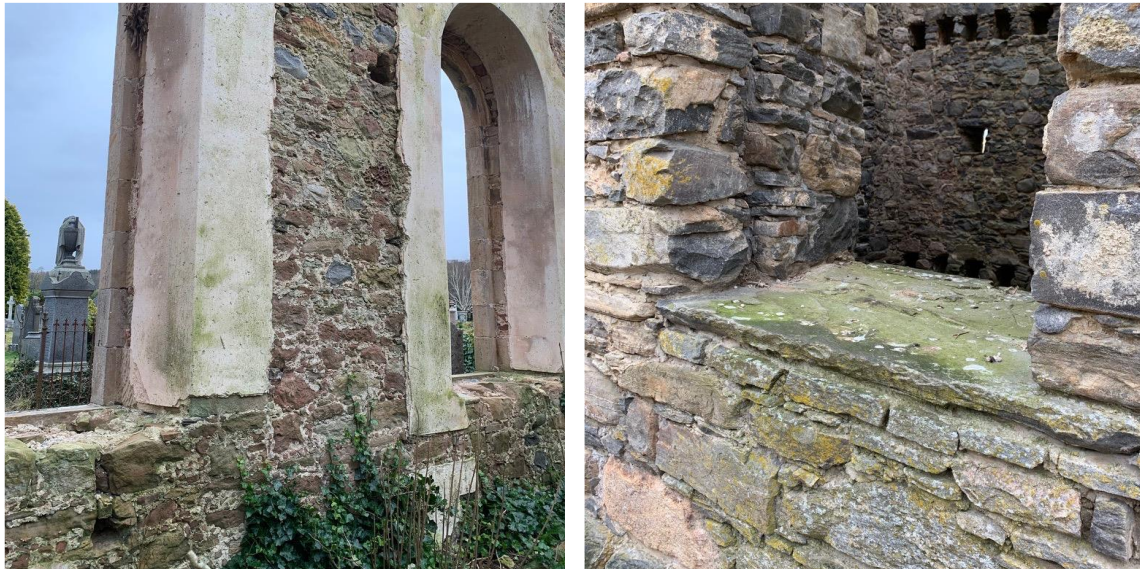
Figure 4.4. Left: the Gaelic Chapel, Cromarty, Ross shire. Right: The Ruthven Barracks, Kingussie. Full width walls where there is no requirement for a view.
