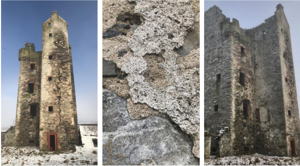
Figure 3.18. Fairburn tower, Inverness shire. Main and Stair towers. Centre the Main Tower FDC mortar overlain with 17 th century Stair Tower harl.
