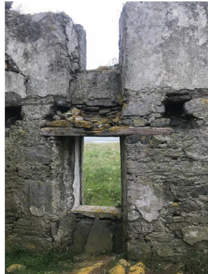
Figure 4.17. Left: Newhall House steadings. Lintel with droved raised face and stugged and broached set-back for harl. Right: Old Vallay House timber safe lintels.
