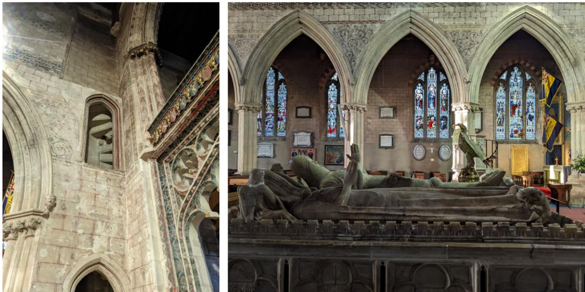
Figure 1.4. St Mary's Church, Berkeley, Gloucestershire, plastered walls with polychromatic illustrations of ashlar. Image credit Imogen Gower.
