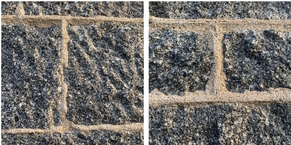
Figure 2.53. Houghton House, raised ribbon pointing: Left the mortar spilling out of the joint. Right: the raised ribbon.
