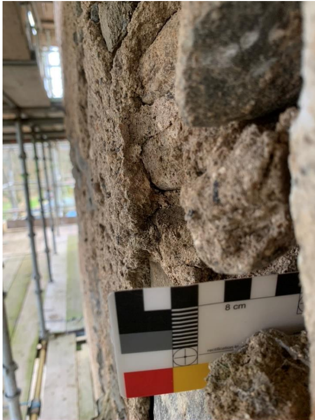
Figure 3.42. FT003 Main Tower, north elevation, sample removed from large structural crack.
