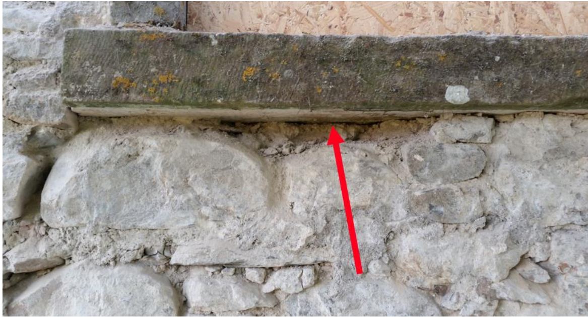
Figure 4.13 Large stone and slate support the sill: where the sill is unsupported a small crack has formed.
