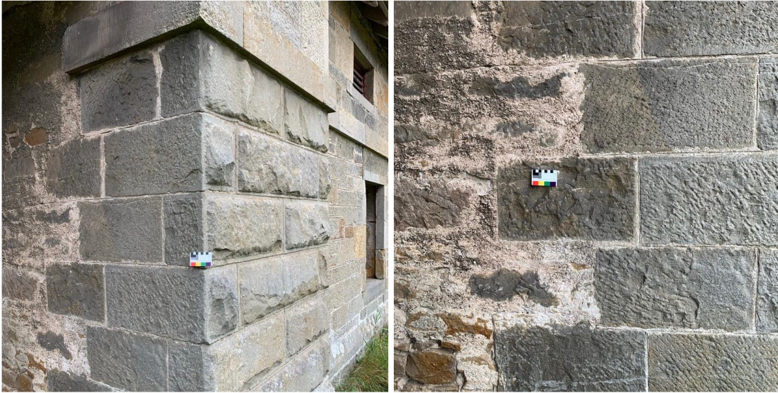
Figure 2.65. The junction where the main front elevation meets the worn harled side.
