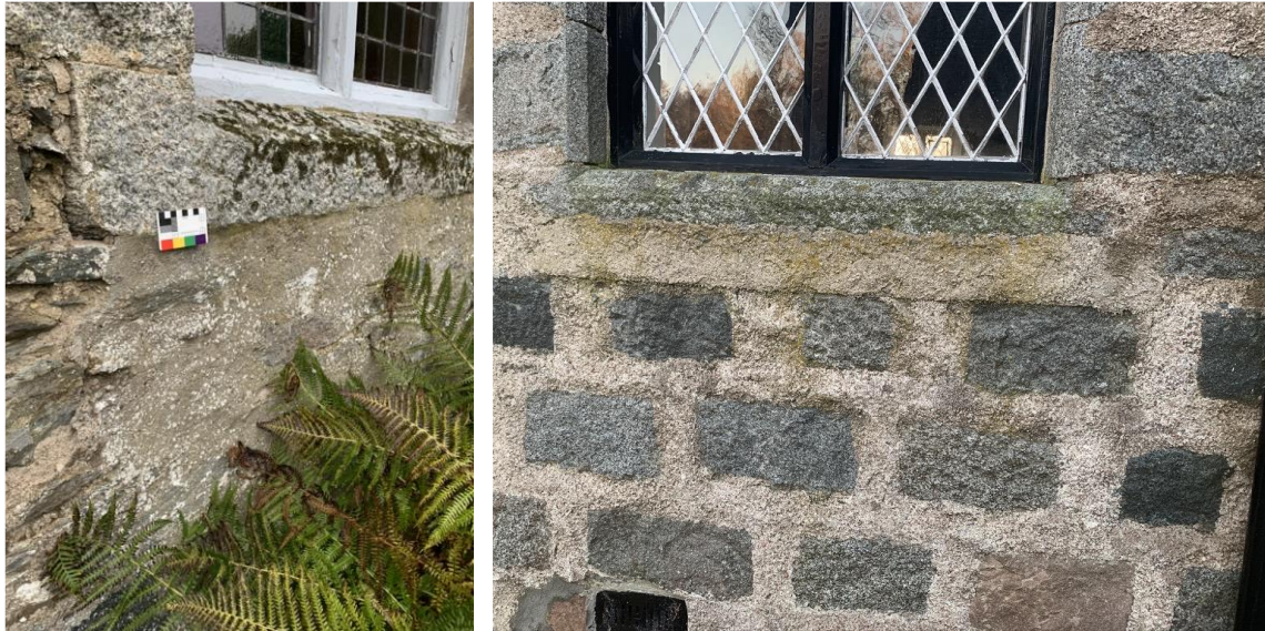
Figure 4.15. Left: St Michael's 7 All Angels Church, Ballintum, Blairgowrie. Right: Deeside Church, Torphins, Aberdeen shire, showing reinforcement to the under-sill areas and additional sneck harl.
