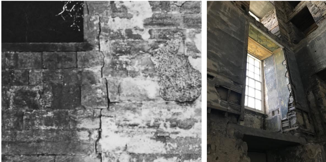
Figure 4.9. Left, detail of the cracking and right a sense of the determination to achieve symmetry despite the wall width.
