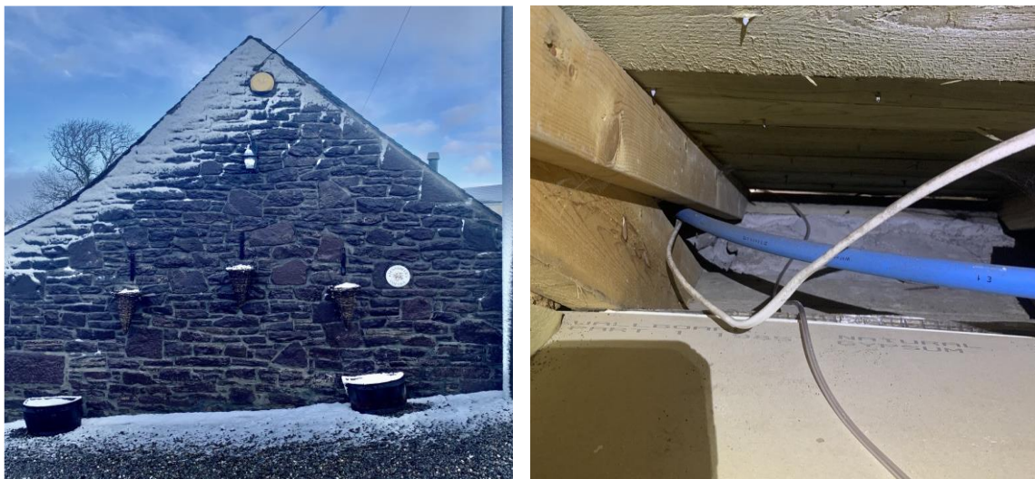
Figure 4.36. Showing the south-west gable of the cottage and the gap between the wall head and underside of the sarking. Note the plastic tube from the manometer directed through the gap to the gable where the pressure readings were taken.
