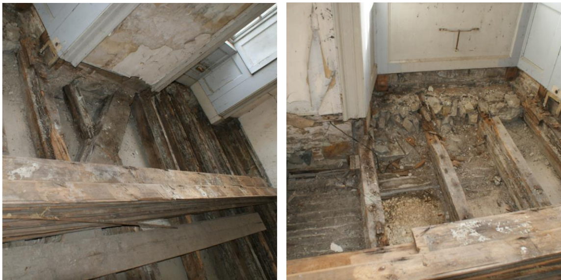
Figure 4.28. The floor joists have decayed after being set into diminished masonry window openings.
