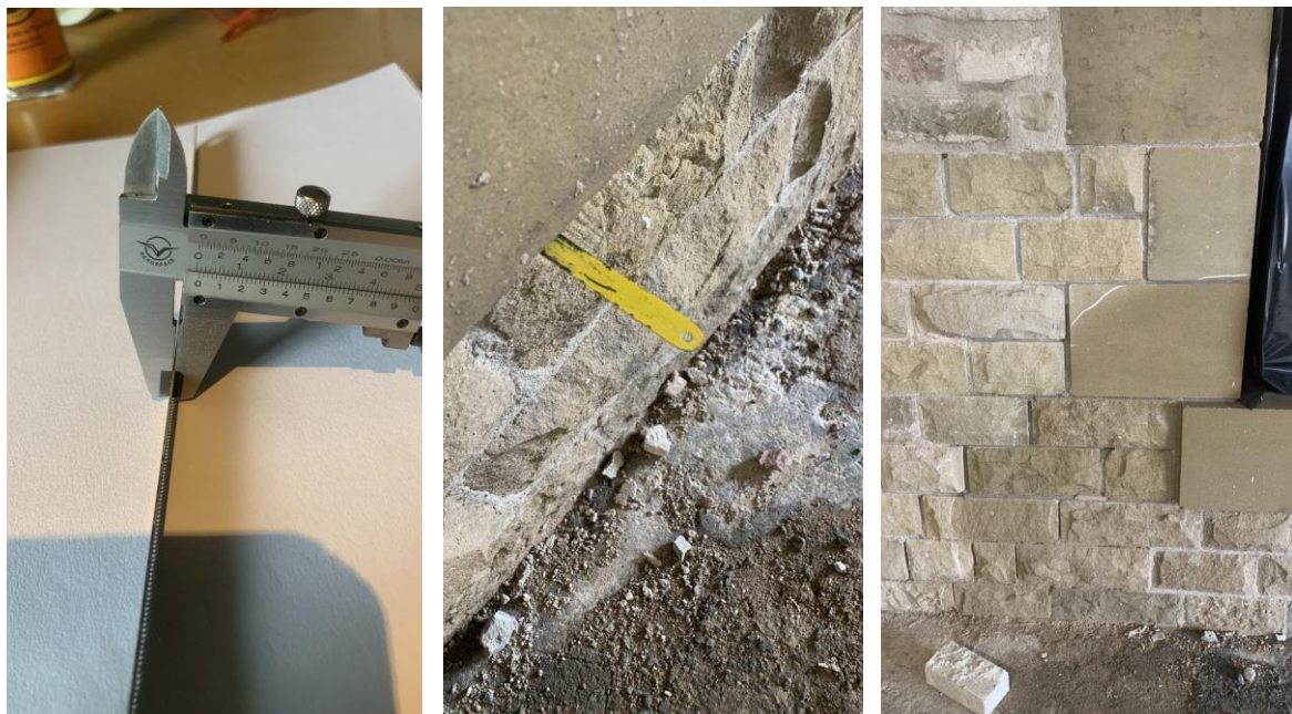
Figure 5.9. Replicating the under-sill crack with manufactured slot using a modified saw blade.
