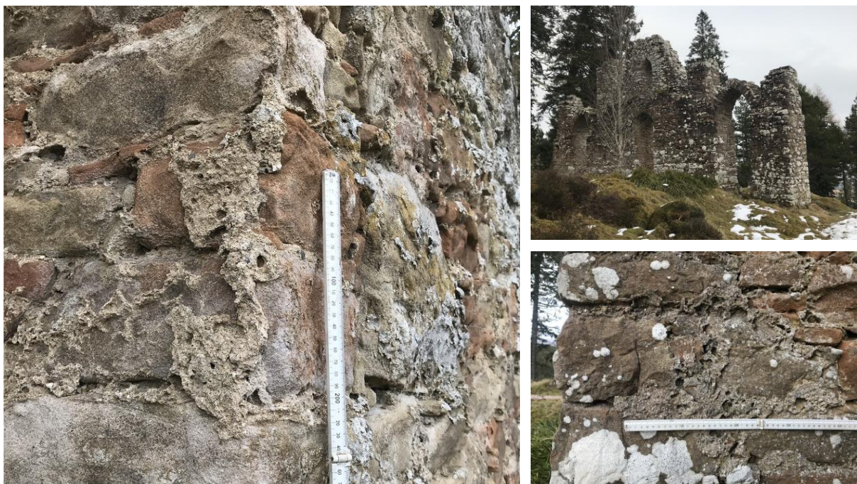
Figure 3.14. The Fryish Monument, c. 1782 Ross shire. Mortar extruded from the joints and remaining on the face of the sandstone, and where the sandstone can be seen weathering.
