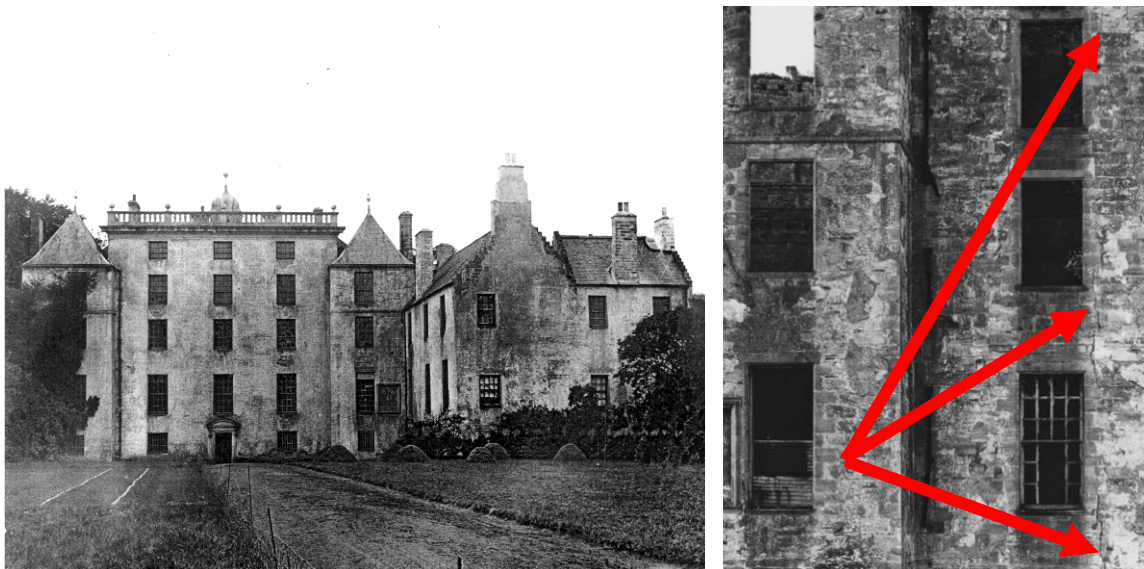
Figure 4.8. Kinniel House, Bo'ness: Left, the 16 th c Main Tower, and additional flanking 17 th c. wings. The symmetrical fenestration of the Main Tower punched through at the same time as the wings. Right, the red arrows indicating the cracking associated with punching through the windows.
