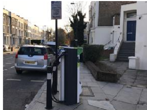
E-taxi charger narrowing footway
