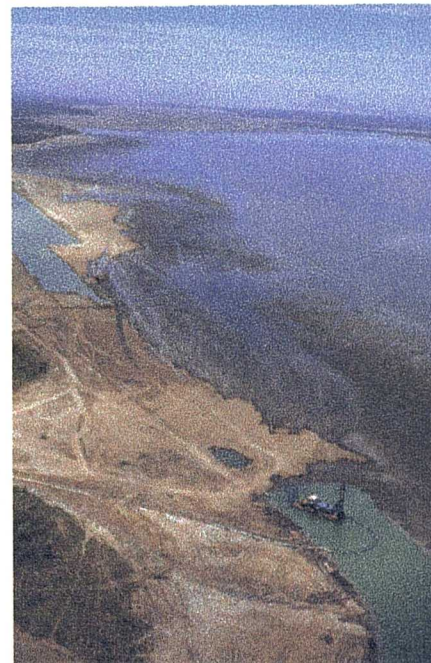
Plate X. Aerial view of a new channel being constructed parallel to the sand barrier in Huizache (17 April, 1995).
