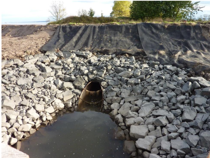
Fig. I-4 Pipe fitted through the sea wall permitting the sea water to enter in the restored site of Skinflats (Forth estuary, UK). Photo: Romuald Rouger
