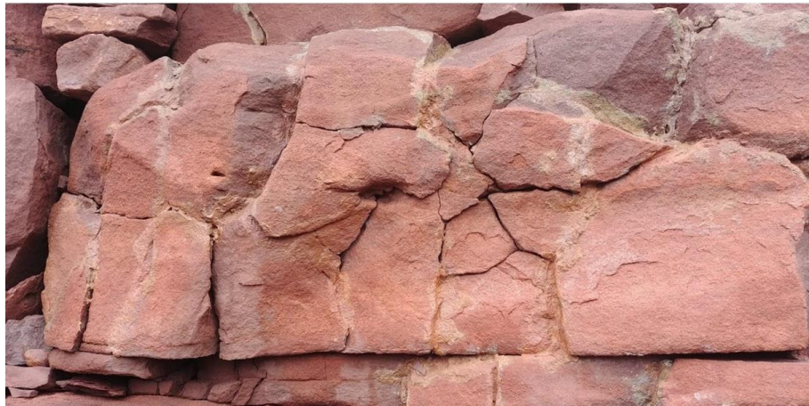
Figure 6.3 - Face bedded block within Clachtoll Broch, showing signs of extensive surface cracking and flaking
