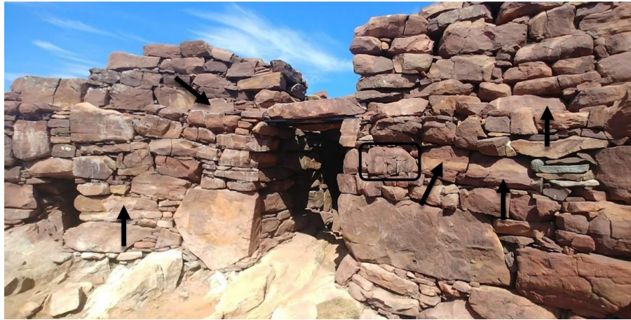
Figure 6.2 - Clachtoll Broch wall face, packing stone sits proud of larger face bedded blocks, some examples of which are highlighted. The block shown in Figure 6.3 is circled
